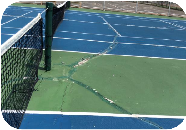
Extensive cracking across courts, lifting of surface and crumbling of base.
