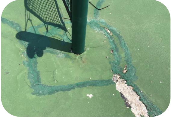
Cracking and damage around net post. Note continued cracking, lifting of surface layer and crumbling of base causing trip hazards.
