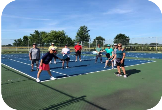
Pickleball Players at Malden Courts. Note darkening of courts in foreground due to wear, uneven surface and water damage. Extensive crack can be seen on left side.
