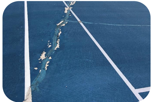
Note peeling of surface from base, crumbling base and indentation of surface. Court has been repaired previously however indentation is visible and darkening of surface shows further damage.
