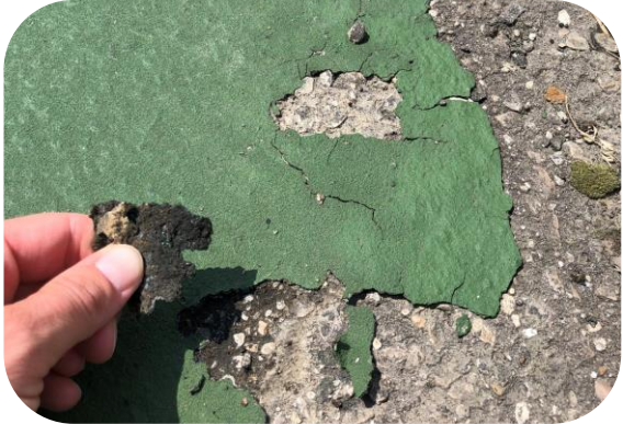
Closeup of lifting of surface and crumbling of base material.
