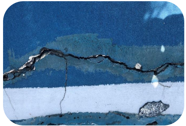
Closeup of extent and width of cracking on a repaired area causing trip hazards.
