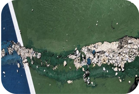
Closeup of peeling and breakdown of base.
