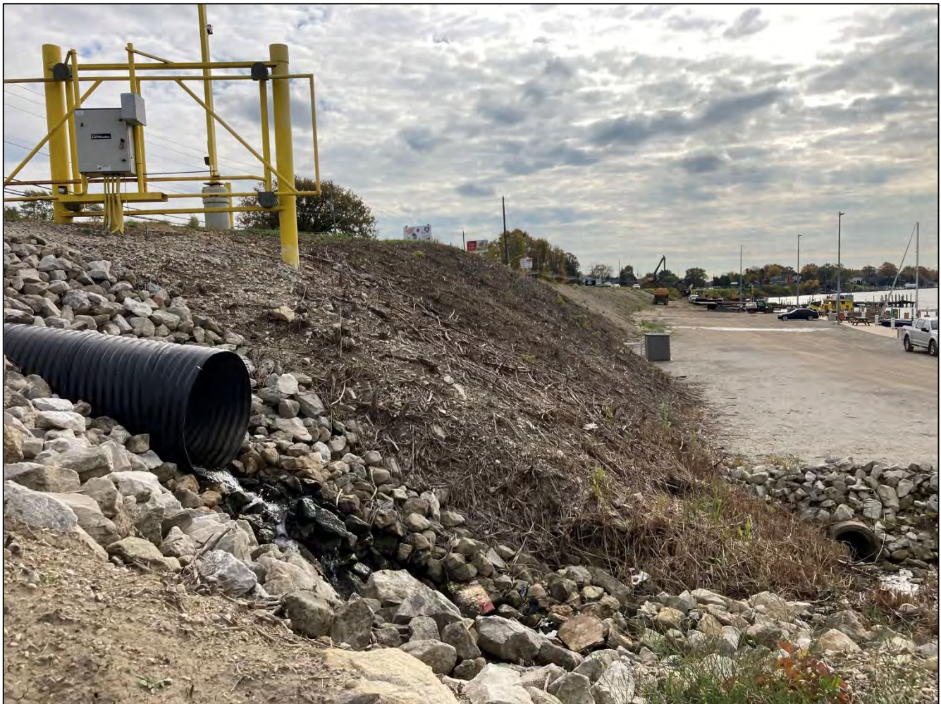
Photo 4: Perched culvert outlet of the artificial drainage ditch at the marina on the Detroit River side of Sandwich Street (04 November 2021).
