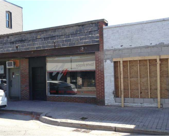
Where possible remove cladding, paint, or other coverings which hide the original brick façade material
