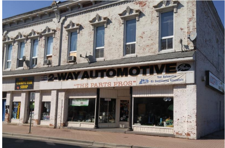
Historical façade in need of restoration 70-72 Murray Street
