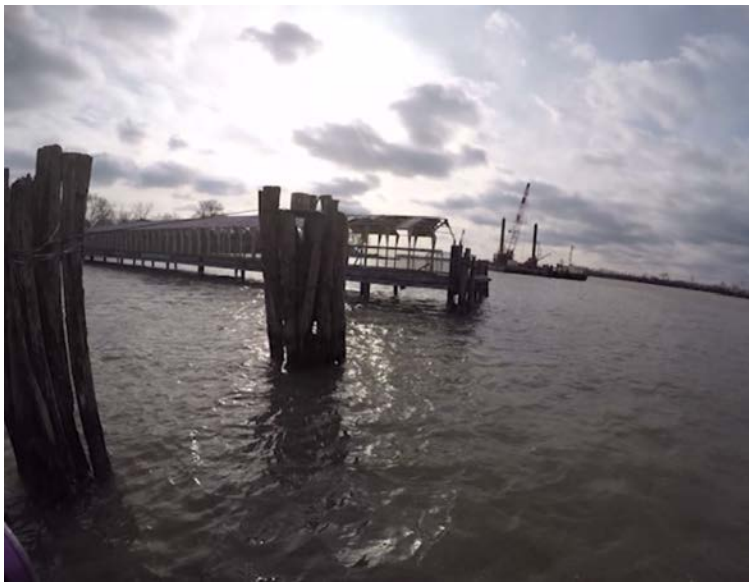
Figure 2-2 View of Northern end of pier looking along bent line 14 toward the South-West.
