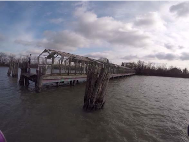
Figure 2-3 View of Northern end of pier looking along bent line 14 toward the North East.
